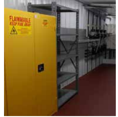
FLAMMABLE SAFETY - STORAGE RACKS AND SHELF WORKSPACE
